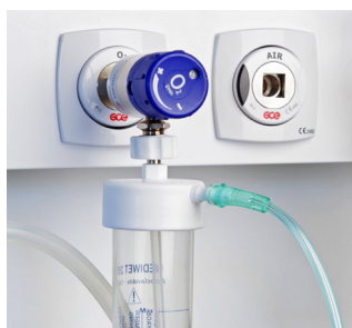
FLOW SELECTOR CONNECTED TO HOSPITAL TERMINAL UNIT
